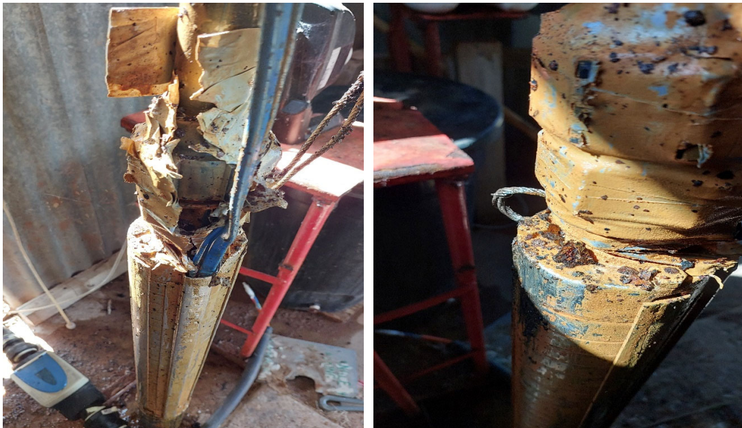
Condition of pumping equipment showing Iron Bacteria and rusted casing pieces.
